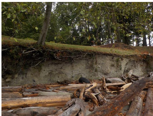
Evidence of shoreline bank erosion due to backshore vegetation losses. Valdes Island - Photo: RC de Graaf
