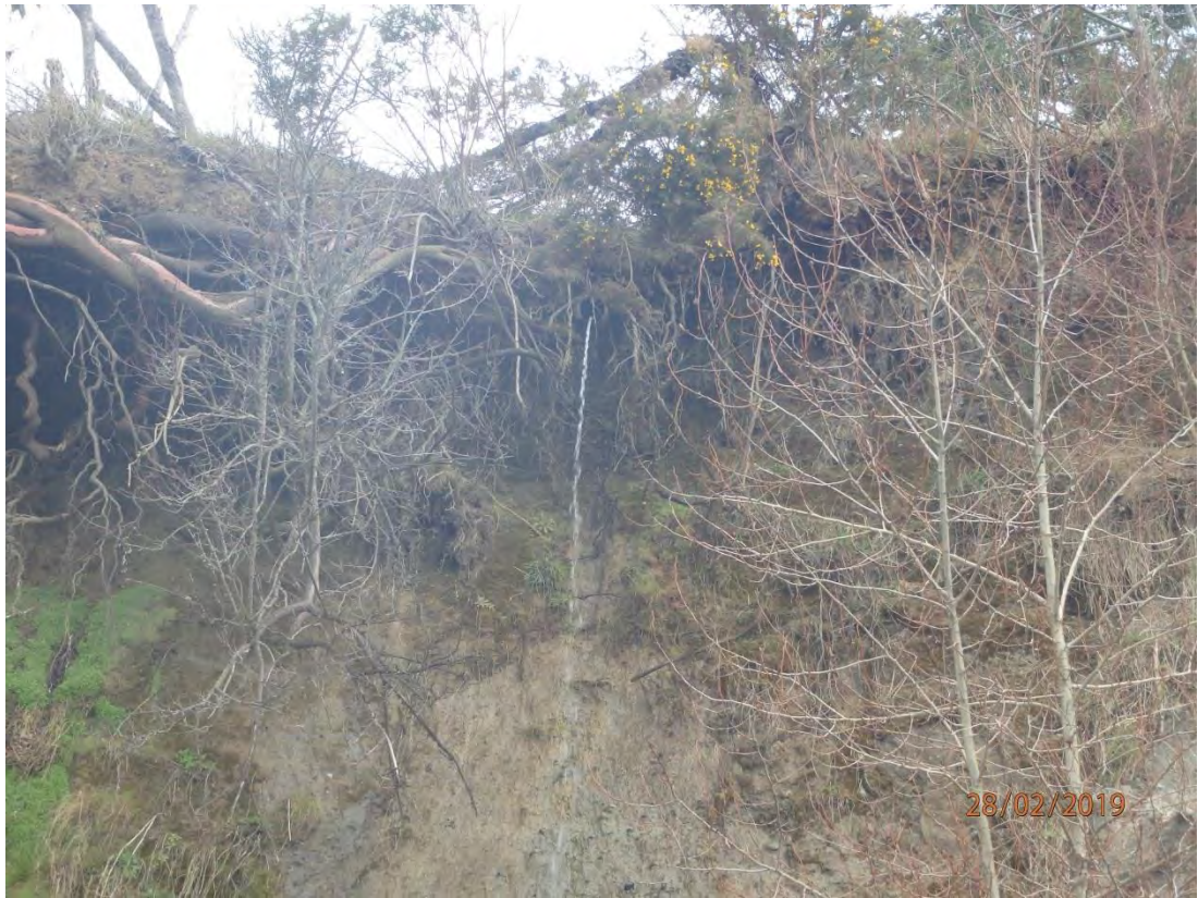
OUTFALL PIPE - BEACH UNIT 11.
