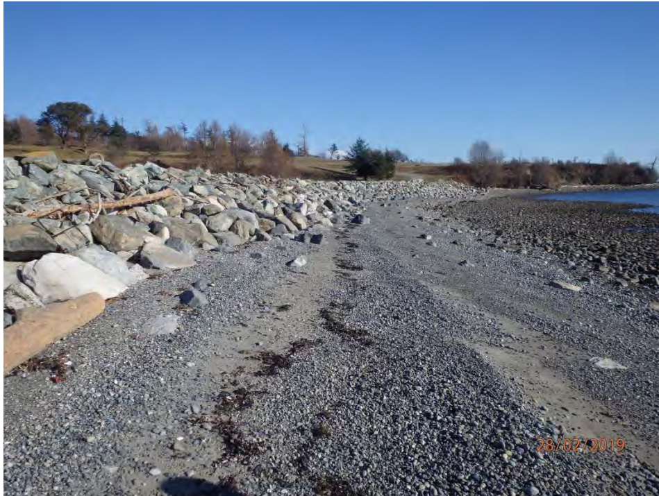
RIP-RAP ARMOURING ALONG THE MAIN JAMES ISLAND ACCESS ROAD LEADING FROM THE DOCK – BEACH UNIT 19.
