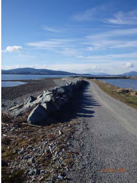
LOOKING NORTH ALONG THE ACCESS ROAD RUNNING ALONG THE SPINE OF THE SAND SPIT (BEACH UNIT 19 IS LOCATED TO THE WEST). NOTE RIP-RAP THAT PROTECTS THE EXPOSED WESTERN SIDE OF THE ROAD.
