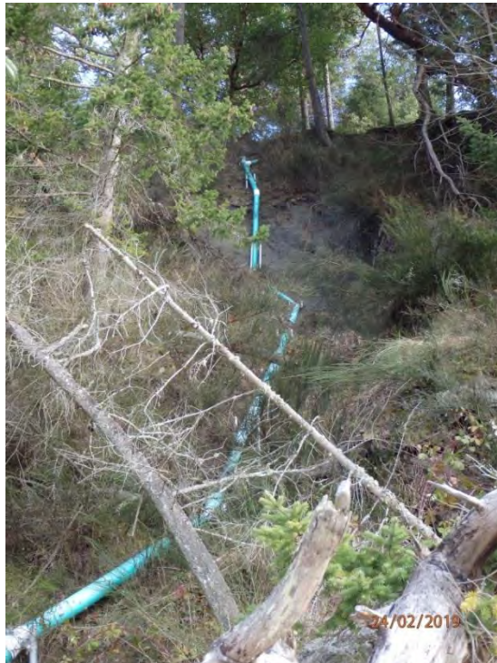
ABOVE AND BELOW: STORMWATER OUTFLOW PIPES PLACED THROUGH THE MARINE BACKSHORE ZONE AND DISCHARGING ONTO THE BEACH – BEACH UNIT 4.
