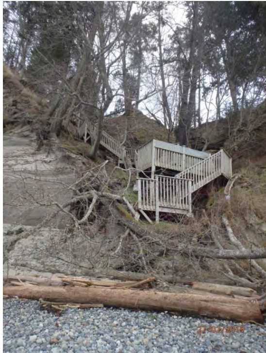
LOOKING WEST TOWARDS A BEACH ACCESS STAIRWAY LOCATED IN BEACH UNIT 29. THIS FEATURE IS CURRENTLY UNUSABLE, BASED ON THE INSTABILITY OF THE SLOPE.
