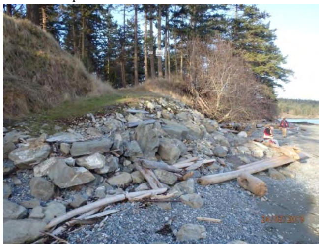
LOOKING EAST TOWARDS THE ACCESS RAMP AND RIP-RAP ENCROACHING INTO THE BACKSHORE ZONE AND FORESHORE AREA – BEACH UNIT 15.
