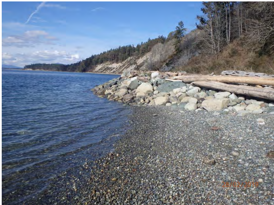
LOOKING NORTH TOWARDS THE RIP-RAP ARMOURING EXTENDING OUT INTO THE FORESHORE AREA ALONG THE EDGE OF THE LANDING SITE IN BEACH UNIT 16.
