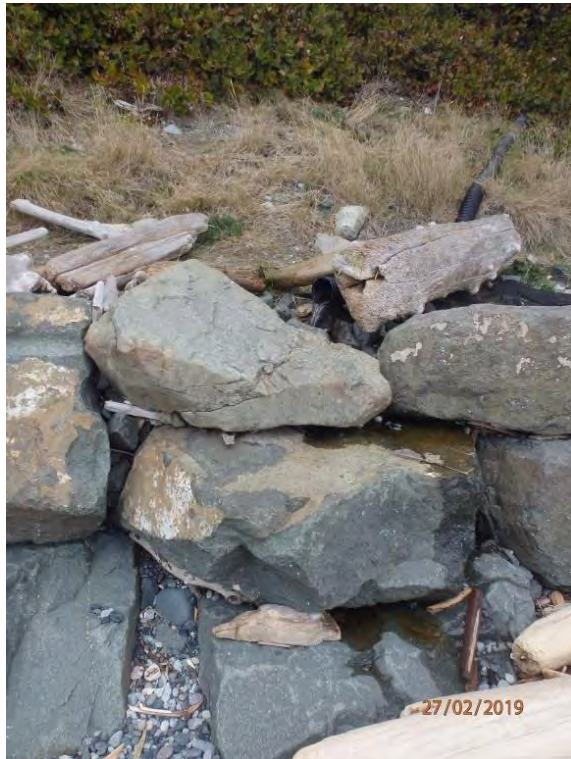
STORMWATER OUTFALL PIPE FLOWING OUT OVER THE RIP-RAP RETAINING WALL LOCATED IN BEACH UNIT 24.
