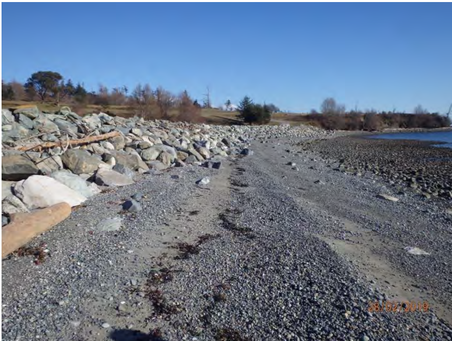
LOOKING SOUTHEAST ALONG BEACH UNIT 19 SHOWING THE RIP-RAP ARMOURING ALONG THE WESTERN SIDE OF THE ACCESS ROAD SHOWN IN THE PREVIOUS PHOTO.
