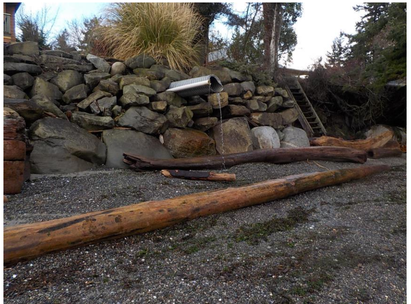
Storm-water outfall pipe, riprap at the high water mark. South coast, Galiano Island Photo: RC de Graaf
